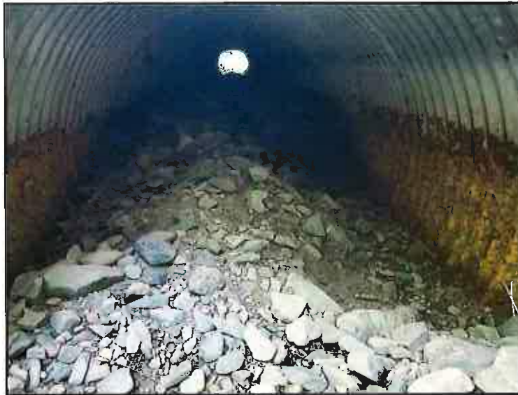
FIGURE 3.3.8 ROCK & SEDIMENT ACCUMULATION – JERRY'S FLAT ROAD MP 8.701
