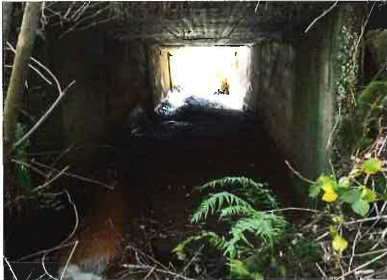
FIGURE 3.3.3 CONCRETE CRACK – PONDEROSA ROAD MP 0.016
