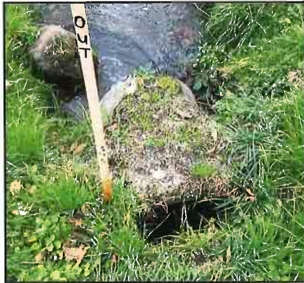
FIGURE 3.3.6 SEPARATED JOINT – WINCHUCK RIVER ROAD MP 0.321
