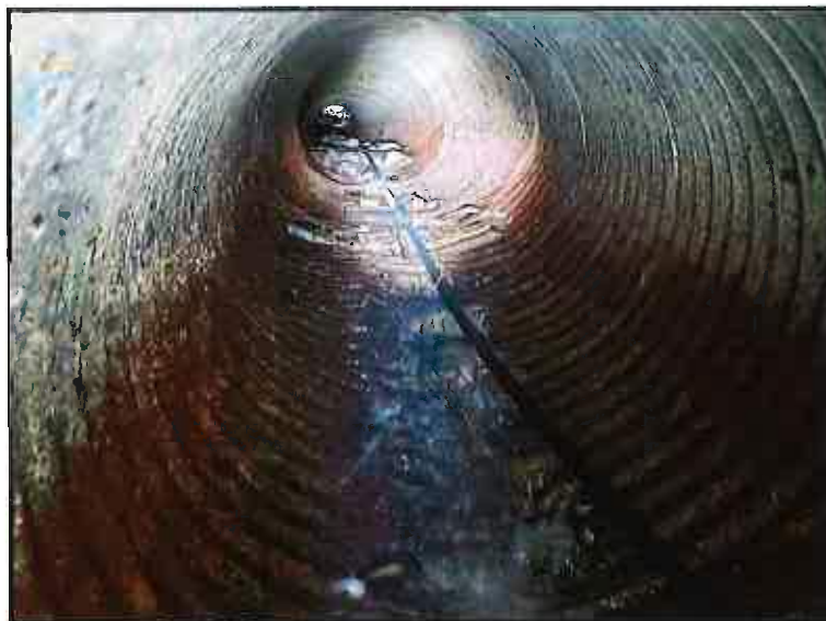
FIGURE 3.3.2 CORRODED PIPE – JERRY'S FLAT ROAD MP 1.955
