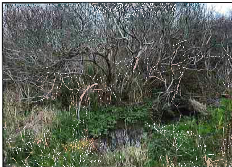
FIGURE 3.5.1 OVERGROWN DRAINAGE PATH TO OCEAN – OLD COAST ROAD MP 0.314
