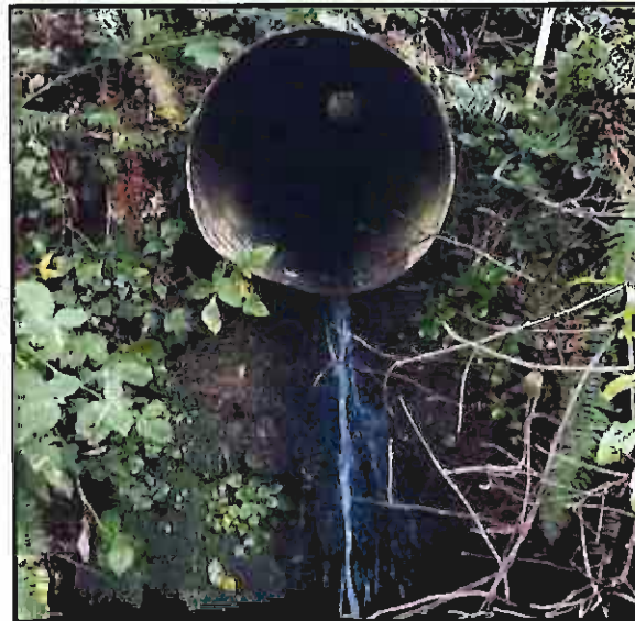
FIGURE 3.3.9 SCOURING AT OUTLET – HILLSIDE ACRES MP 0.299
