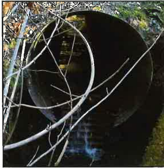
FIGURE 3.3.1 BOTTOM OF CULVERT RUSTED OUT – OAK FLAT ROAD MP 2.41
