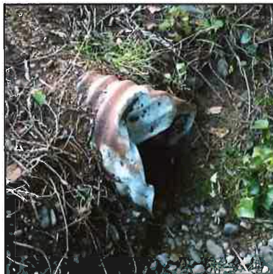
FIGURE 3.3.5 CRUSHED END – SILVER BUTTE ROAD MP 0.137
