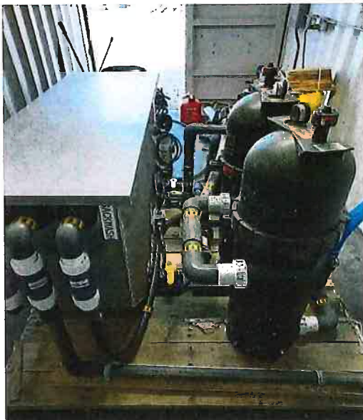
Photo 2. Wash Water Recycle System
