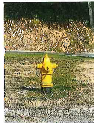
Photo 4. Fire Hydrant at Basin II
