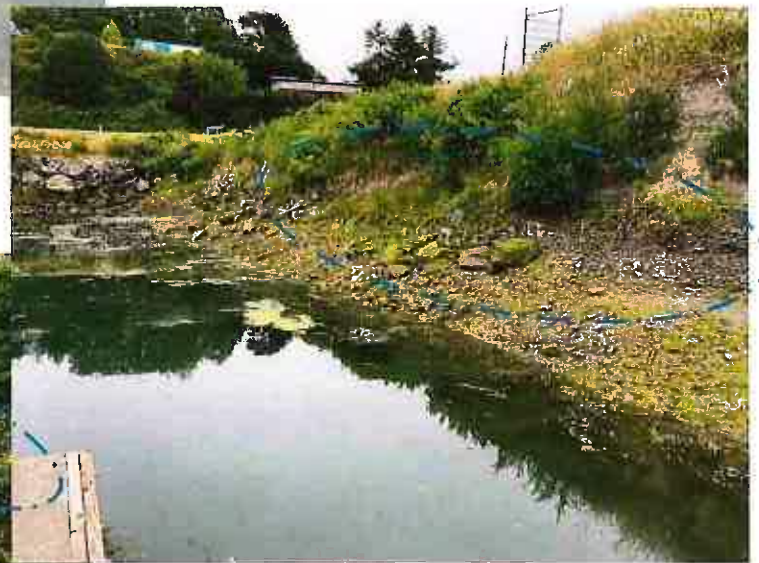
Undersized rock undermined and buried by surge scour during 2019 storms. Note heavier rock, placed with nonwoven fabric at far southeast corner, remains in tact.
