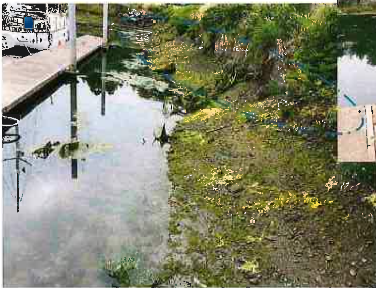
Extreme and abrupt surge scour, caused by amplified storm waves, pulled away and unraveled undersized rock, undermining above embankment. Note young vegetation now overtopping damage.
