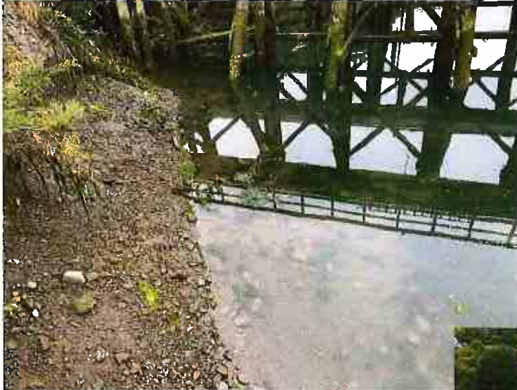
Surge scour during 2019 and subsequent storms are characteristic of end-of-basin damages at the Port of Brookings Harbor.
