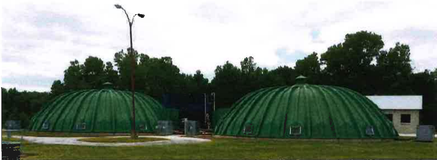
Northern Moraine Utility Commission, Wisconsin – Dome Covered Package Plants Retrofitted with Fixed Biofilm Media
