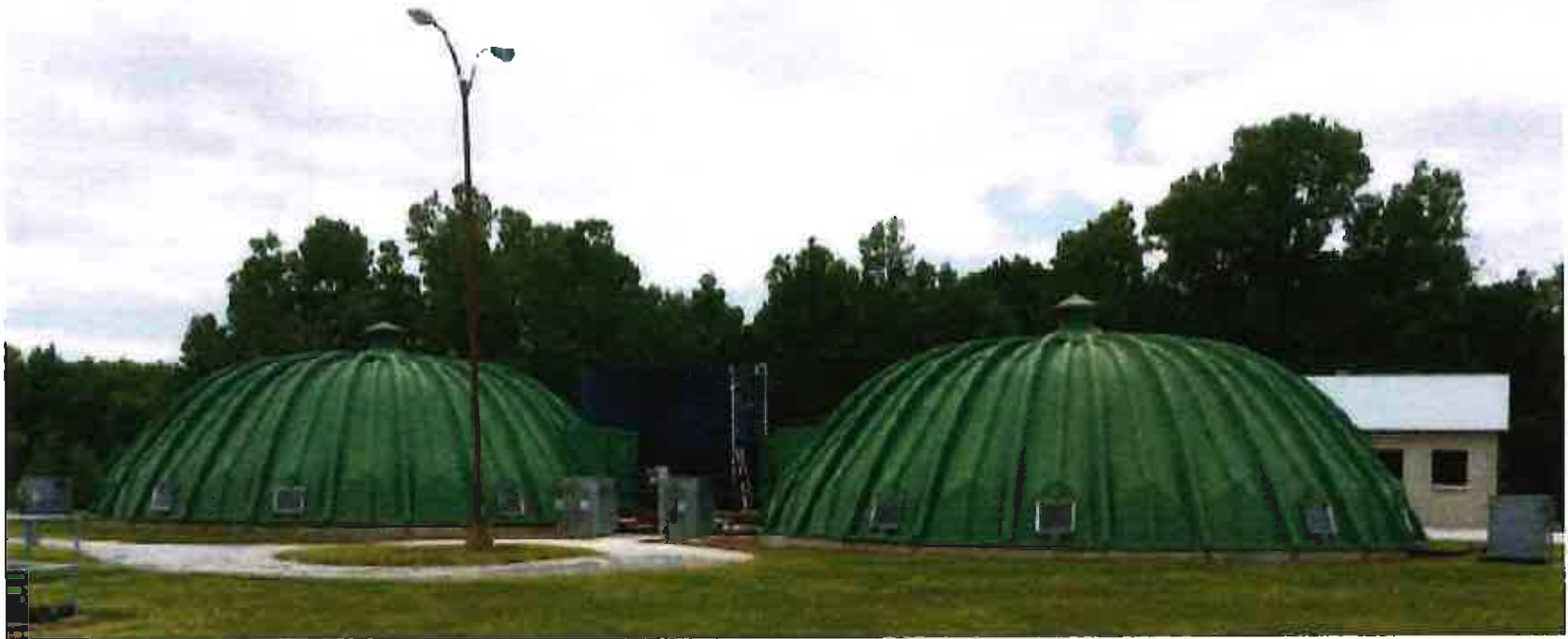
Northern Moraine Utility Commission, Wisconsin – Dome Covered Package Plants Retrofitted with Fixed Biofilm Media
