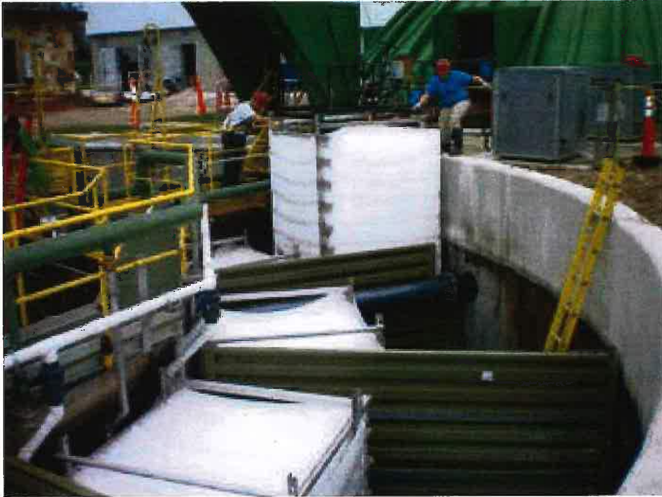
MultiStage Fixed Biofilm Media Installation
