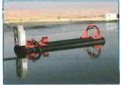
A Mud Cat MC 100E cleans out a water treatment facility pond in Israel.
