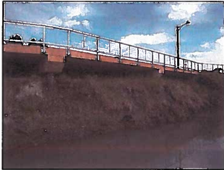
Photo 6 - Falling slope below boardwalk addition
