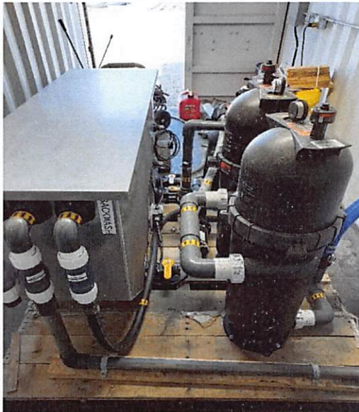
Photo 2. Wash Water Recycle System
