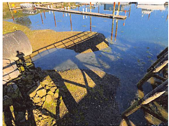
Photo 5. Sediment Impacts to Travel Lift
