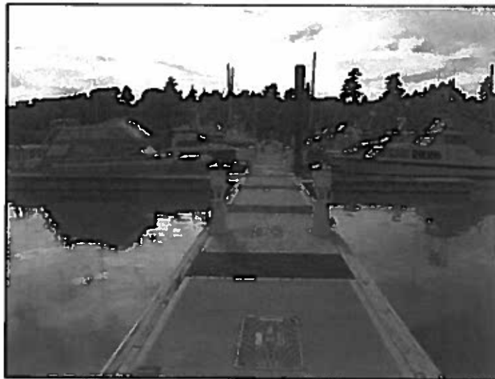
Photo 3 - Power available at sport basin dock
