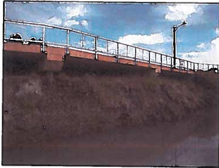
Photo 6 - Falling slope below boardwalk addition
