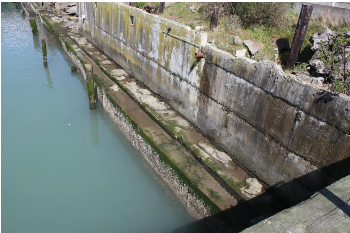
PHOTO 2: Seawall with Scour Beneath Footing
