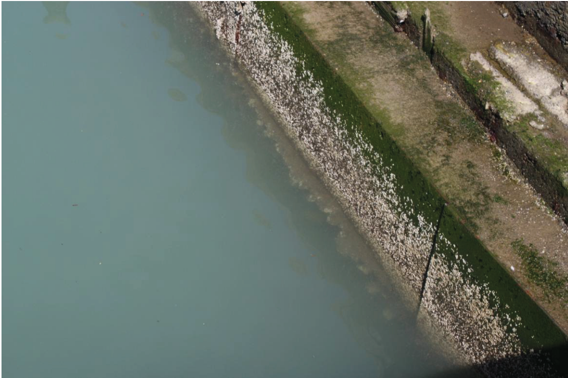
PHOTO 1: Note Undermining of Footing
