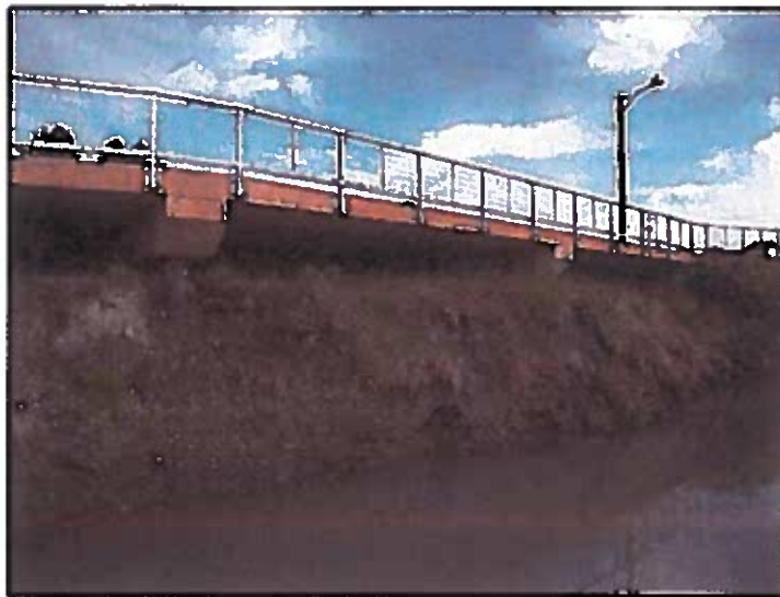
Photo 6 - Falling slope below boardwalk addition
